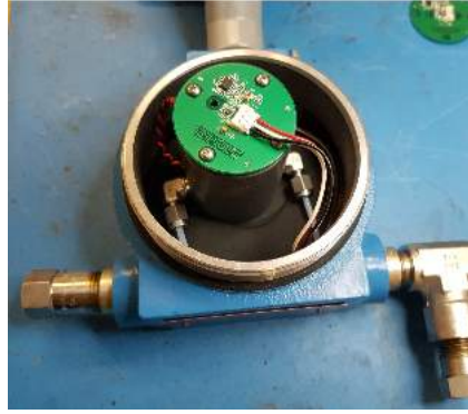
Figure 12: replaced ppm sensor with all fitting and screws tighten.
